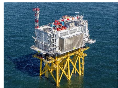
Borssele Beta - installed
